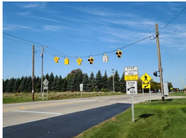
Figure 7: The photo above shows the new HAWK pedestrian crossing on Pine Road between Youngs Ditch Rd looking North to Ridge Road in Hampton Township. This is the very first HAWK signal used in Bay County.
