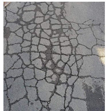
Figure 5: Section of asphalt showing alligator cracking, indicating poor surface condition in need of repair.
